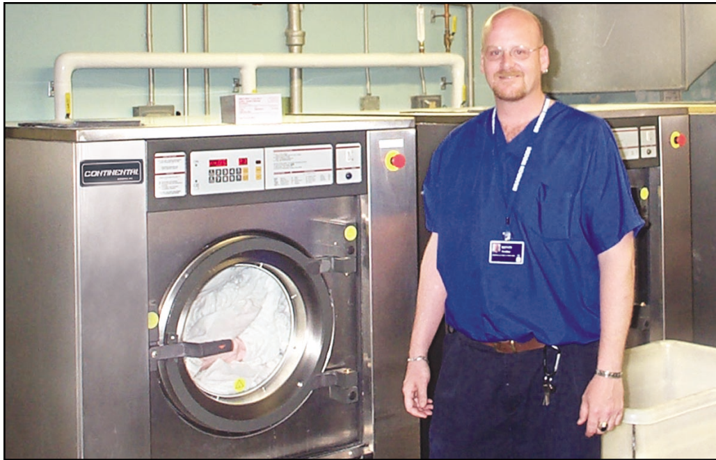
Kevin Svedine, director of housekeeping and laundry, has been pleased with the results since replacing Brandon Woods' laundry equipment with Continental Girbau washer-extractors and dryers. "We're not double-washing, because clothes come out clean the first time," he says.
