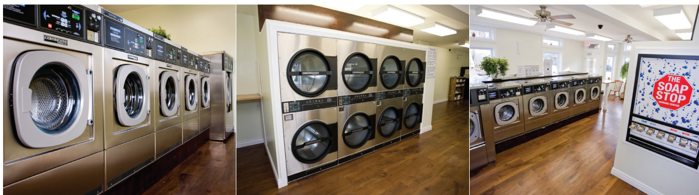
The Eco Laundry Room is a uniquely 'green' laundry complete with solar tubing to heat the store's water; environmentally friendly insulation; T8 florescent lighting; a recycled rubber floor that mimics hardwood; and energy-efficient E-Series Washer-Extractors and Drying Tumblers.
