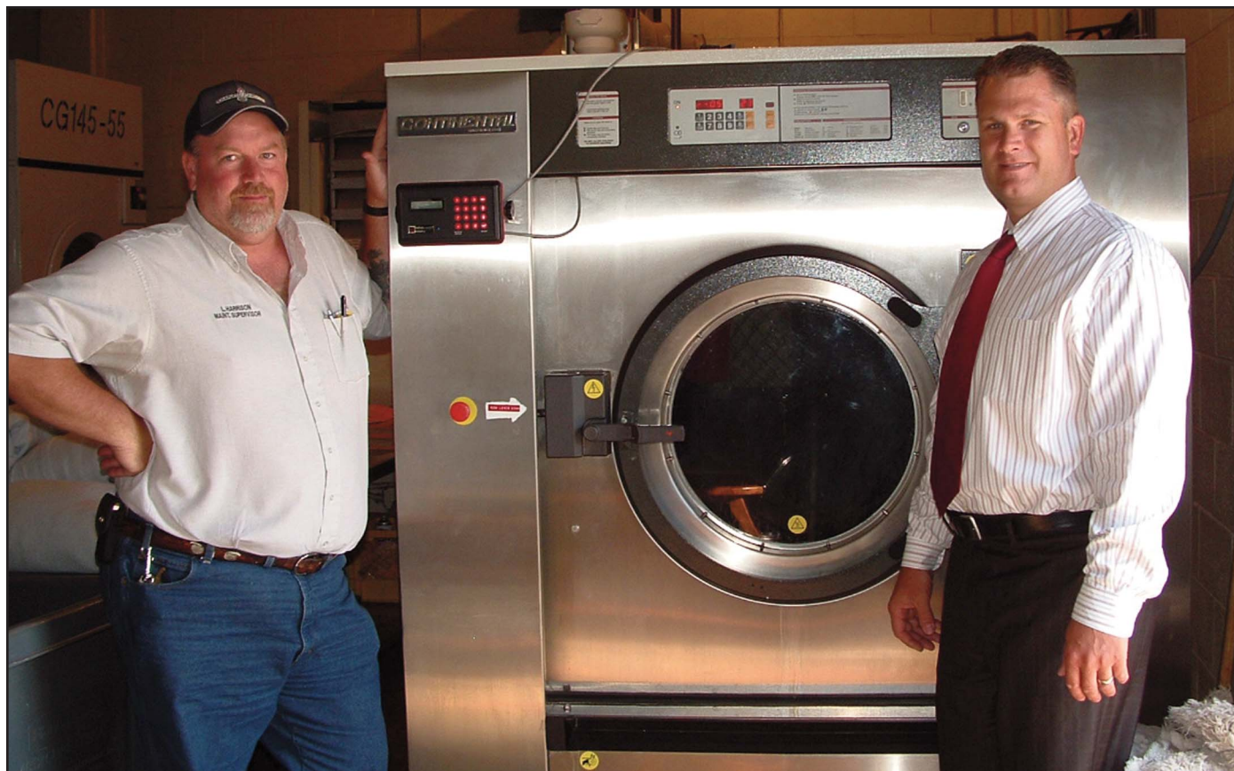
Municipal Correctional Institution's Continental washer-extractors cut their wash time in half. Here, Laundry Room Manager Larry Harrison and Bruce Kusgen, president of All Pro Laundry Equipment are shown in front of the facility's 130-pound Pro-Series Washer-Extractor.
