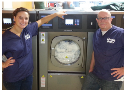
A laundry attendant, left, and Jeff Gardner, right, stand alongside a new on-premise Continental E-Series Washer. Gardner installed the on-premise washer for its superior programmability.
