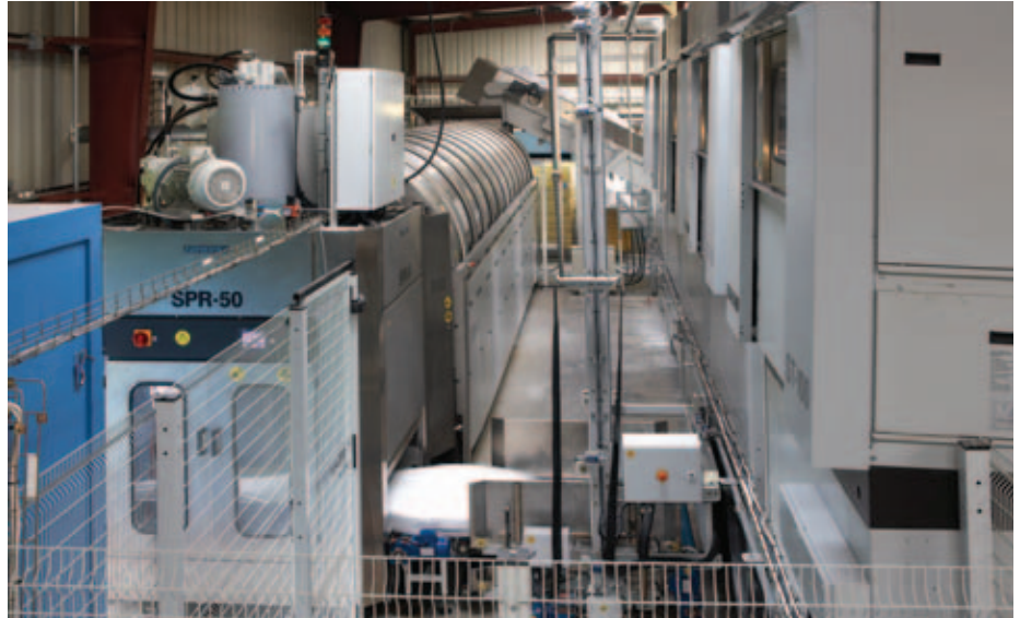
The installation of a Girbau Industrial TBS-50 Continuous Batch Washer helps Laundry Plus keep up with demand during peak season.
