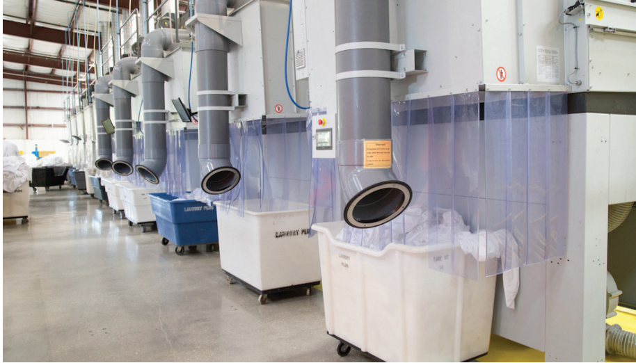
Five of the ST-100 Dryers offer optional vacuum loading for use with the conventional, open-pocket washers. To use the vacuum-loading feature, they are put into manual mode once the tunnels are shut down for the day.
