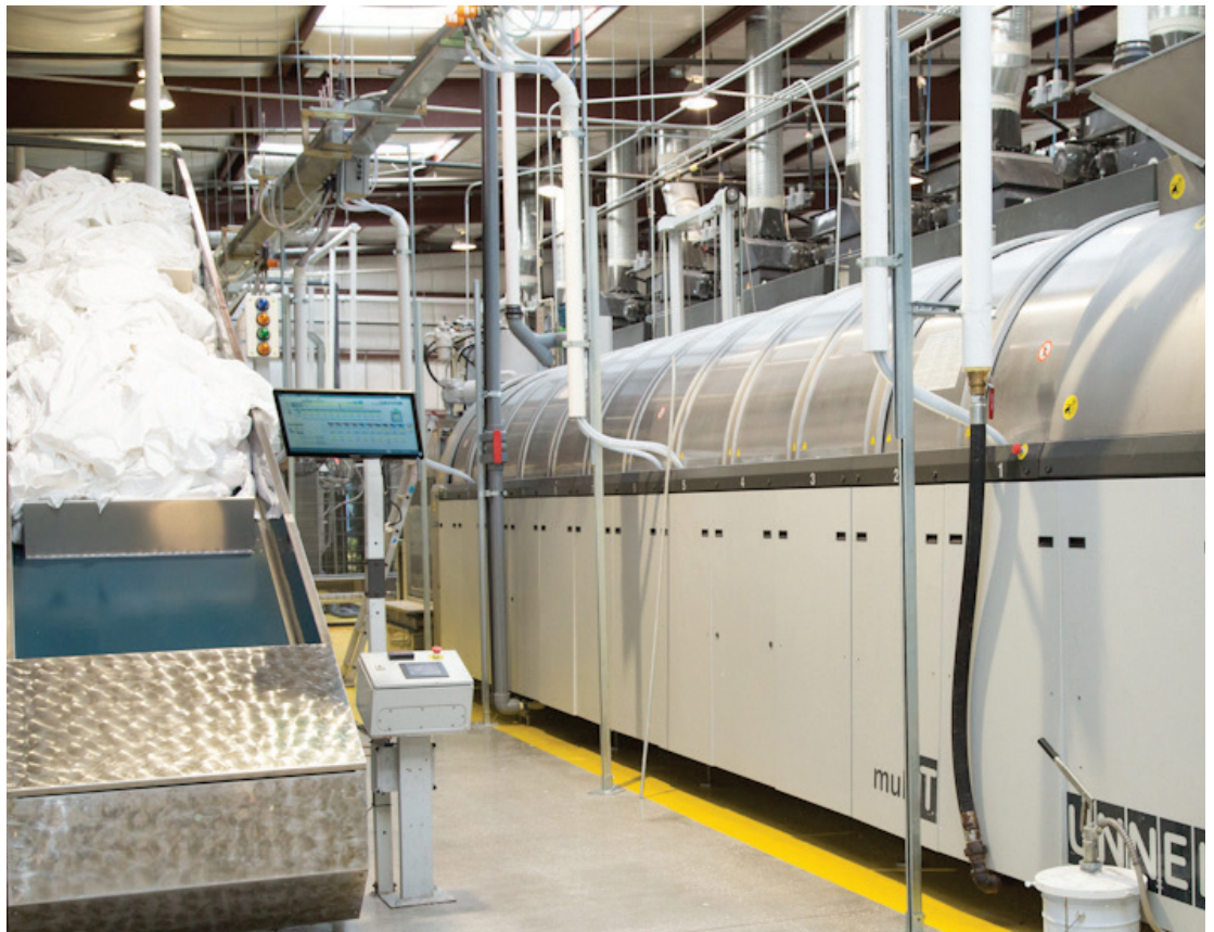
Each of the two GI TBS-50 Batch Tunnel Washing Systems uses shuttles to feed goods into 10 in-line dryers. Rather than each tunnel system having its own dryers, the two are linked to utilize all available dryers. This offers an added bit of protection for Laundry Plus in case one of the tunnels or presses breakdown. Laundry Plus would still be able to utilize all 10 dryers.
