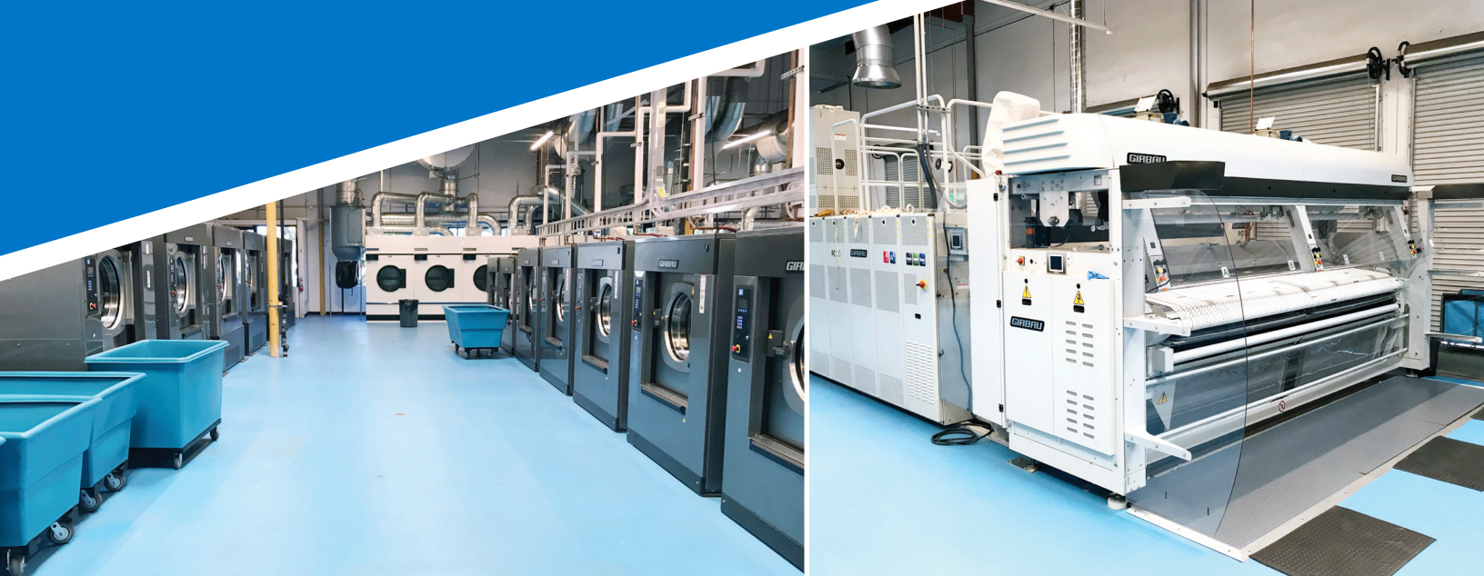
GI washers and dryers handle all incoming laundry at Revolve. Soon, a tunnel system will be installed to up production further.
