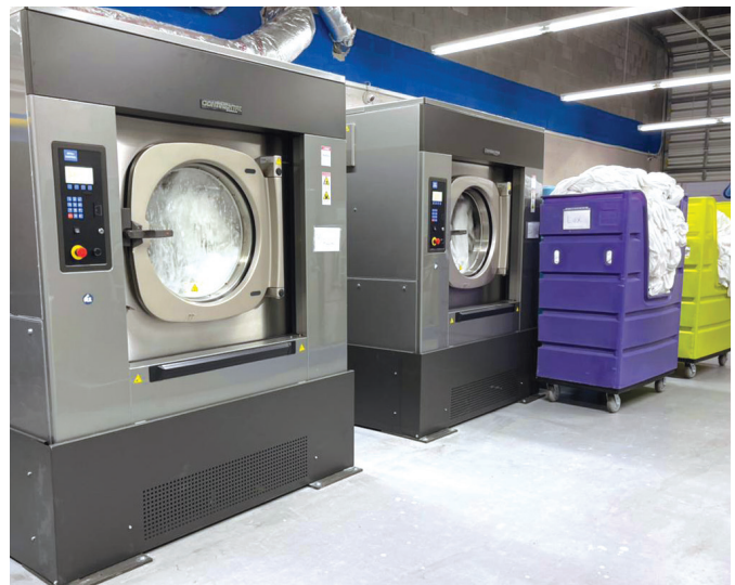
Two GI 255-pound washer extractors were installed to keep up with SerClean’s quick growth.
